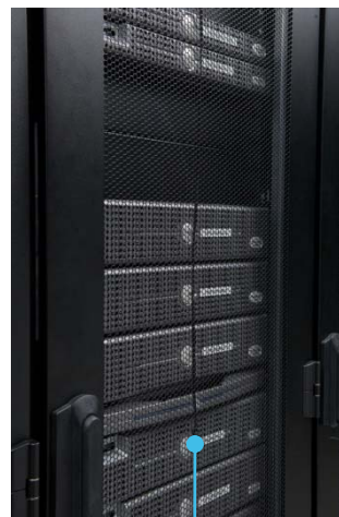
Rack sensors ensure the correct amount of cold air is provided to eliminate hot spots.
