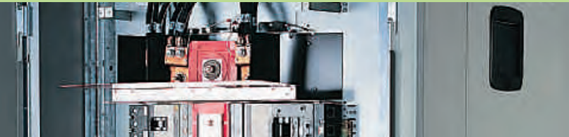
Power Conversion And Distribution
