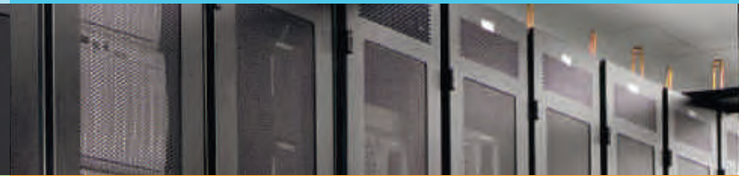
Integrated Racks And Cabinets
