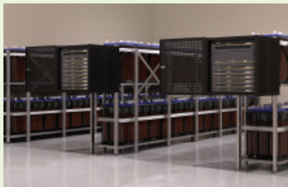
Alber BDS-256XL Monitors and Reports on the Health of Wet Cell Batteries
